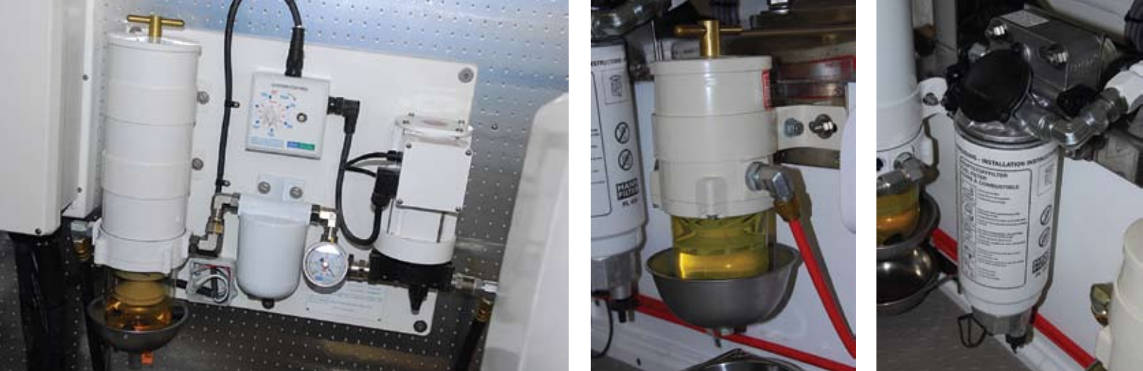
ESI fuel polishing system can polish fuel from any of the four tanks. (top left) Generator primary fuel filters use highly-effective Racor Turbine design. (top center) Additional engine primary filter provides triple filtration. (top right) High-volume fuel transfer pump can move fuel between any two tanks. (bottom)
