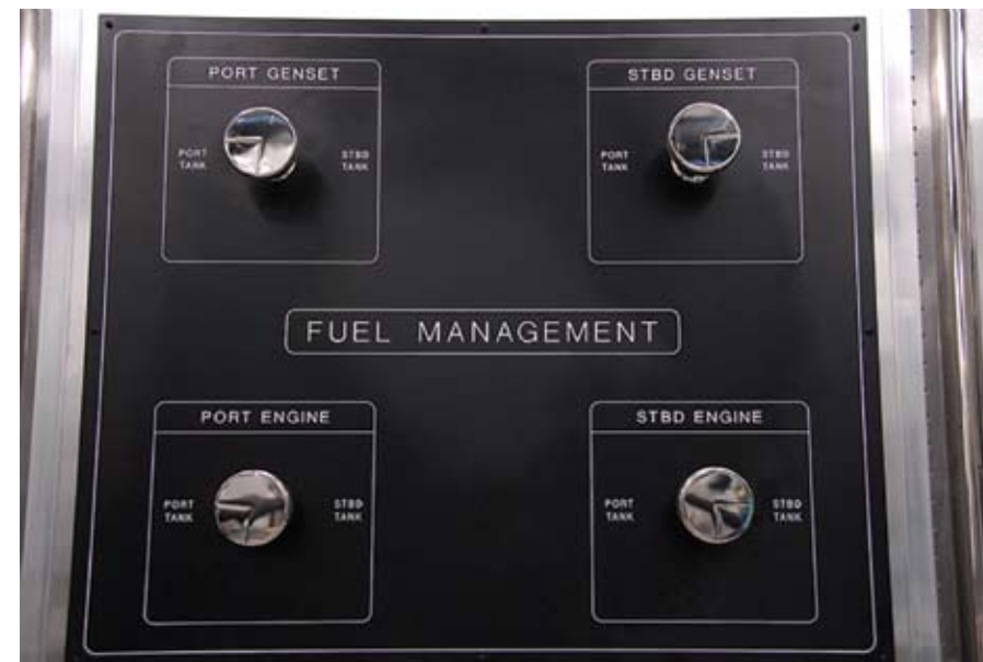
Supply and return valves are synchronized to prevent returning fuel to wrong tank.
